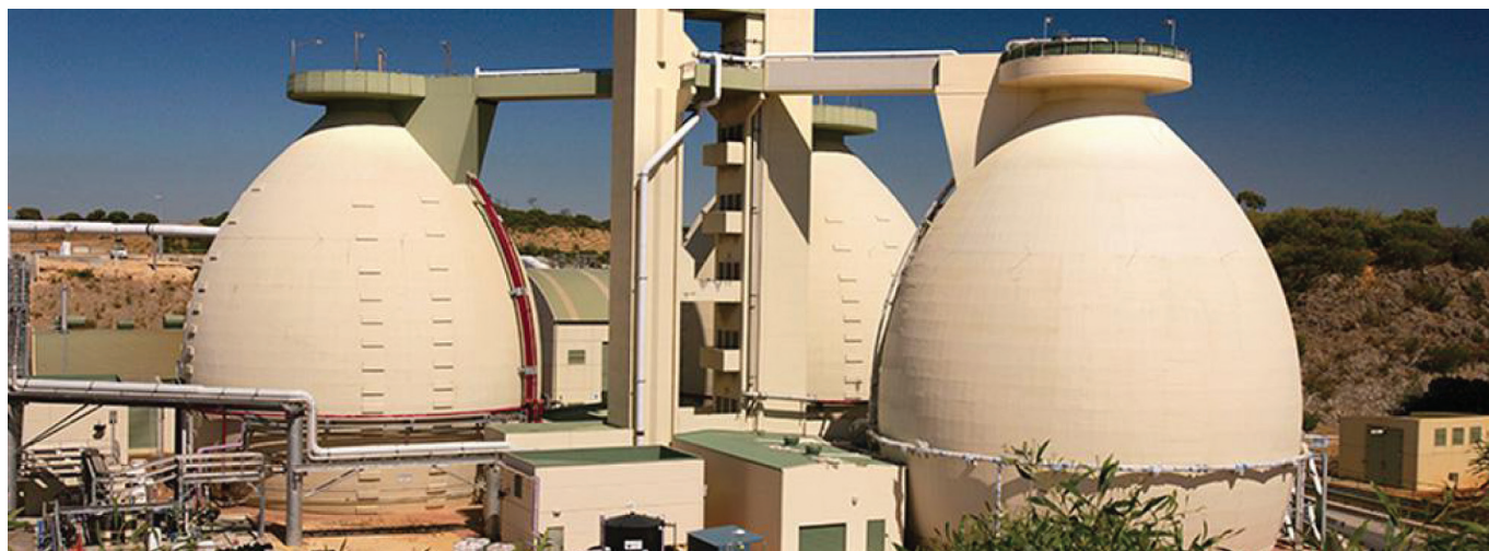
Figure 2. Egg-shaped digesters at Woodman Point WWTP. At 38 metres high, they are the largest of their type in the Southern Hemisphere.
